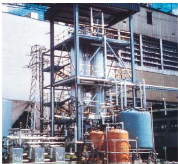
LOPROX® plant, La Felguera, Spain
